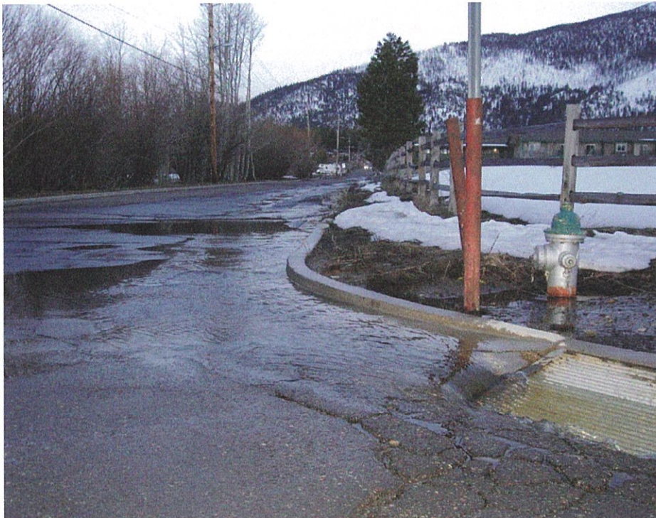
Existing stormwater issues on Kahle Drive
